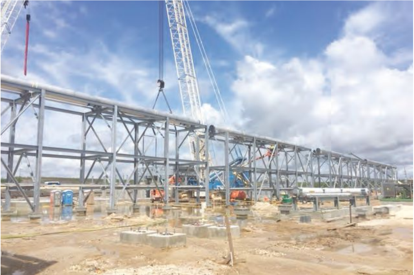
Figure 2: Modular pipe racks being erected at site. The alignment of the foundations is extremely important in such cases as a mismatch would directly result in misaligned pipes at the interface. Note the gaps between the pipes in the module. A make-up piece is field-welded in the gap and takes care of any site tolerances.
