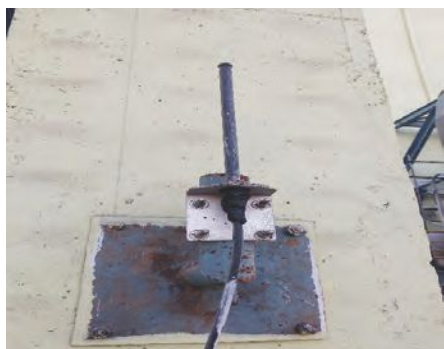
Figure 7: Wireless Antenna Transmitter
